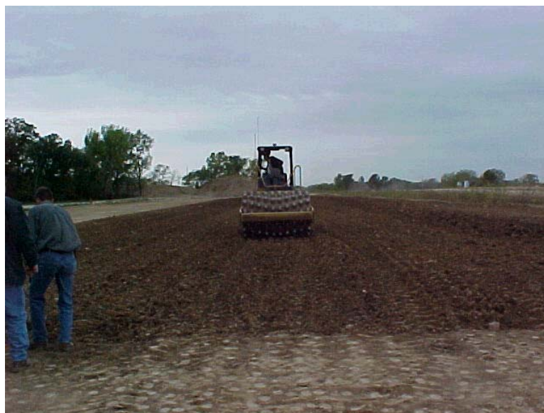
Figure 68: Compaction being performed by CAT CP533E roller in reverse for test strip 2A
